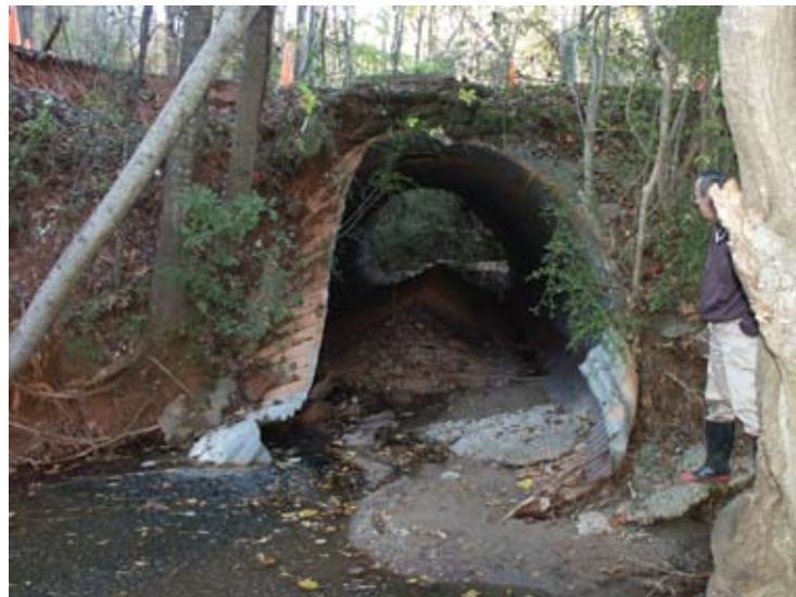
Failing Pipe in Troup County
