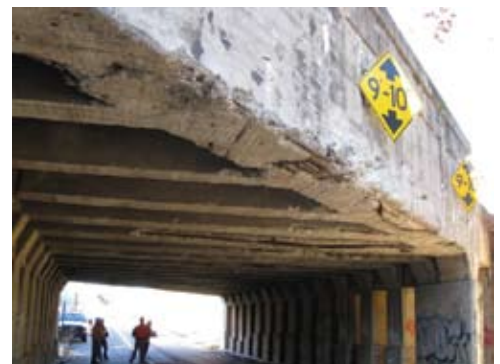
Atlanta bridge in need of repair
