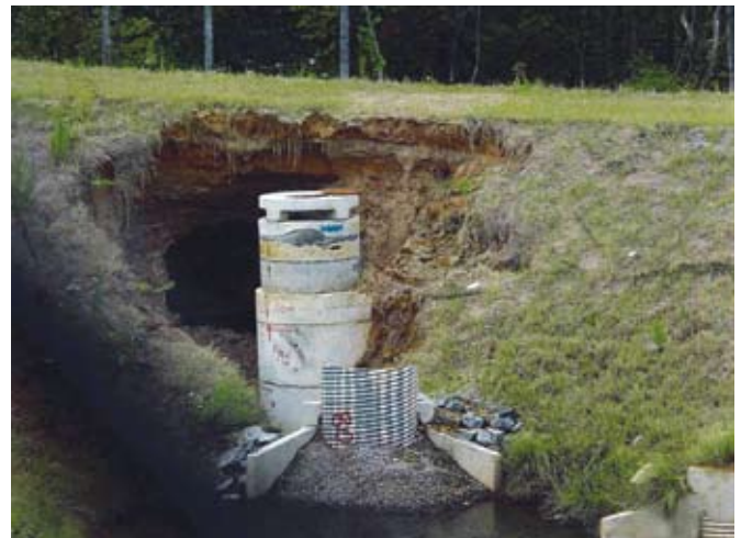
Failure of a dam at an outlet structure
